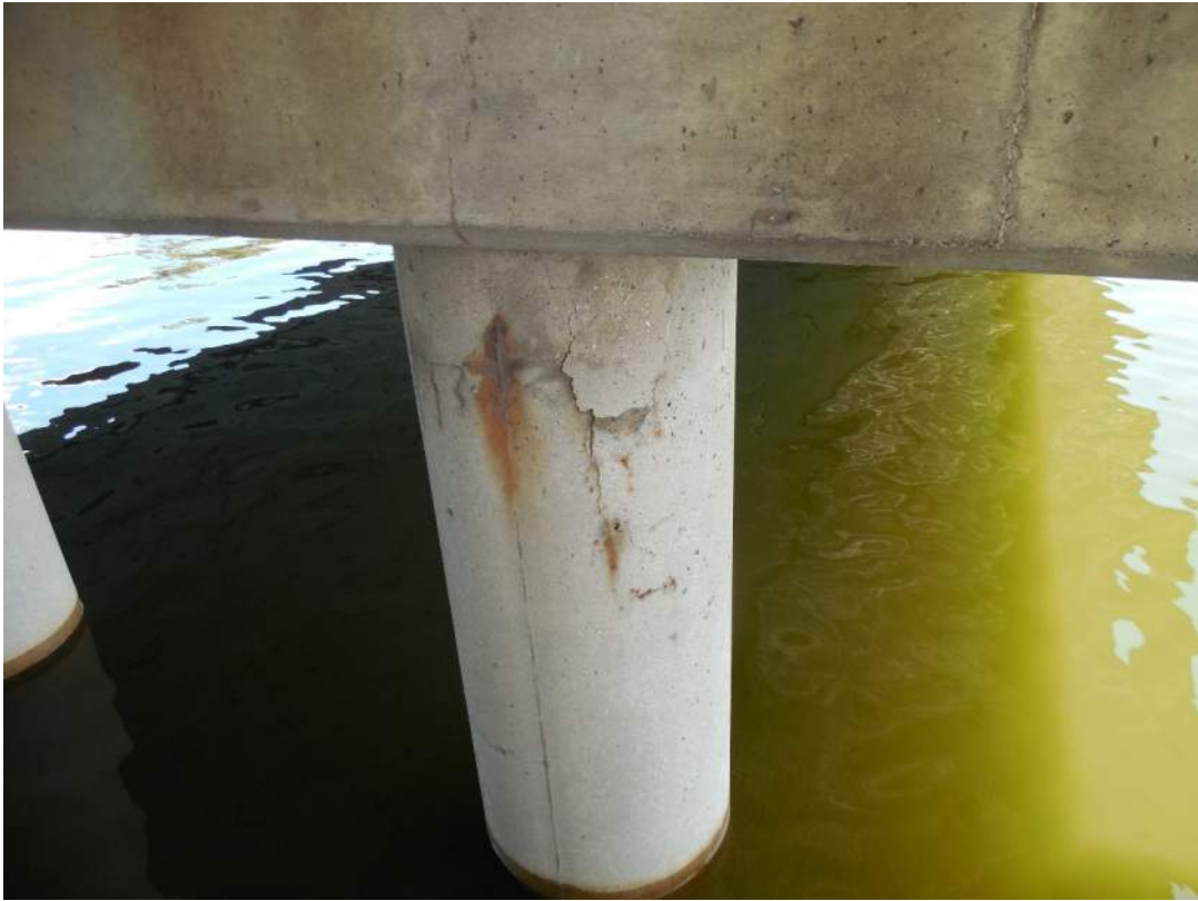
Pier 5S, south face, cracking and delamination on jacket of Pile 5W
