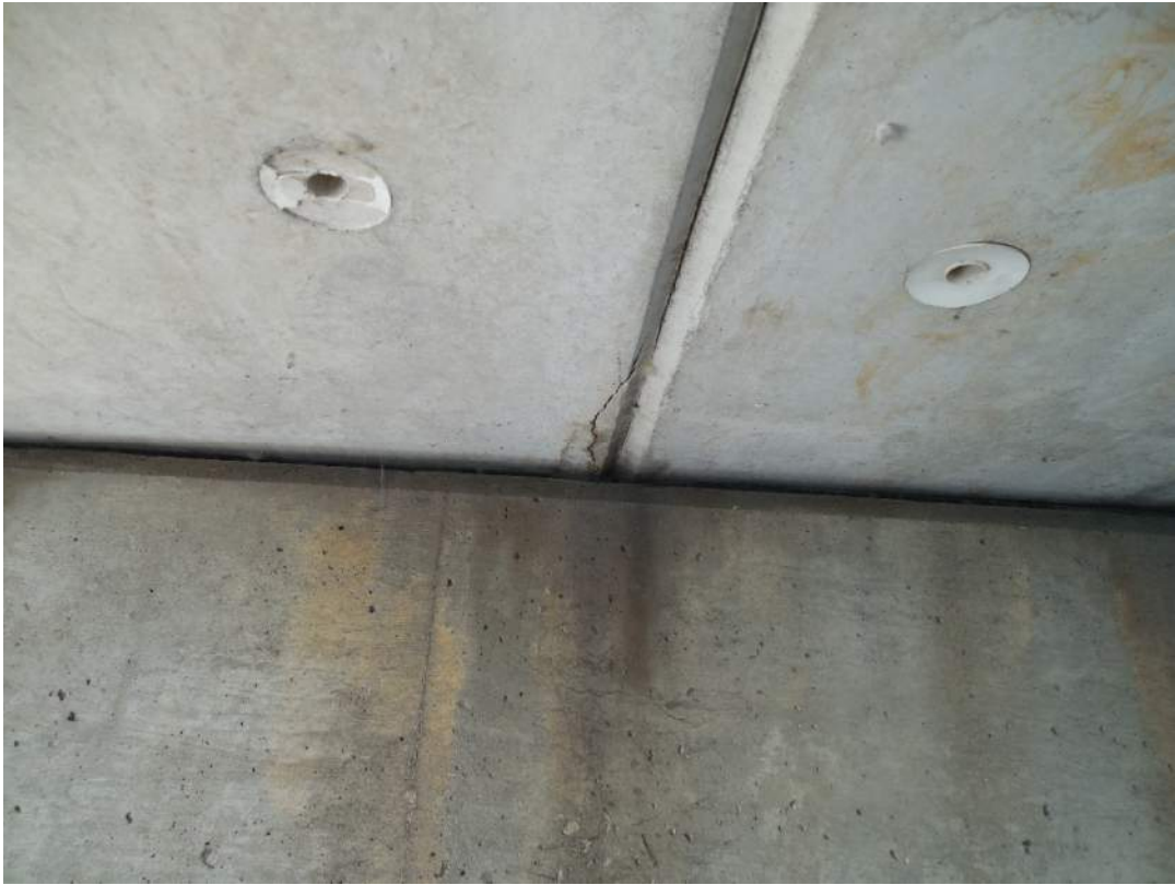
Span 6S, Beam 12W, cracking and delamination at Pier 5S
