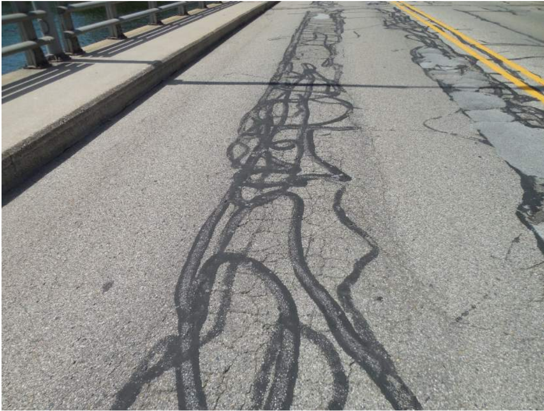
Partially sealed alligator cracking in northbound wheel line, south half of structure, looking south
