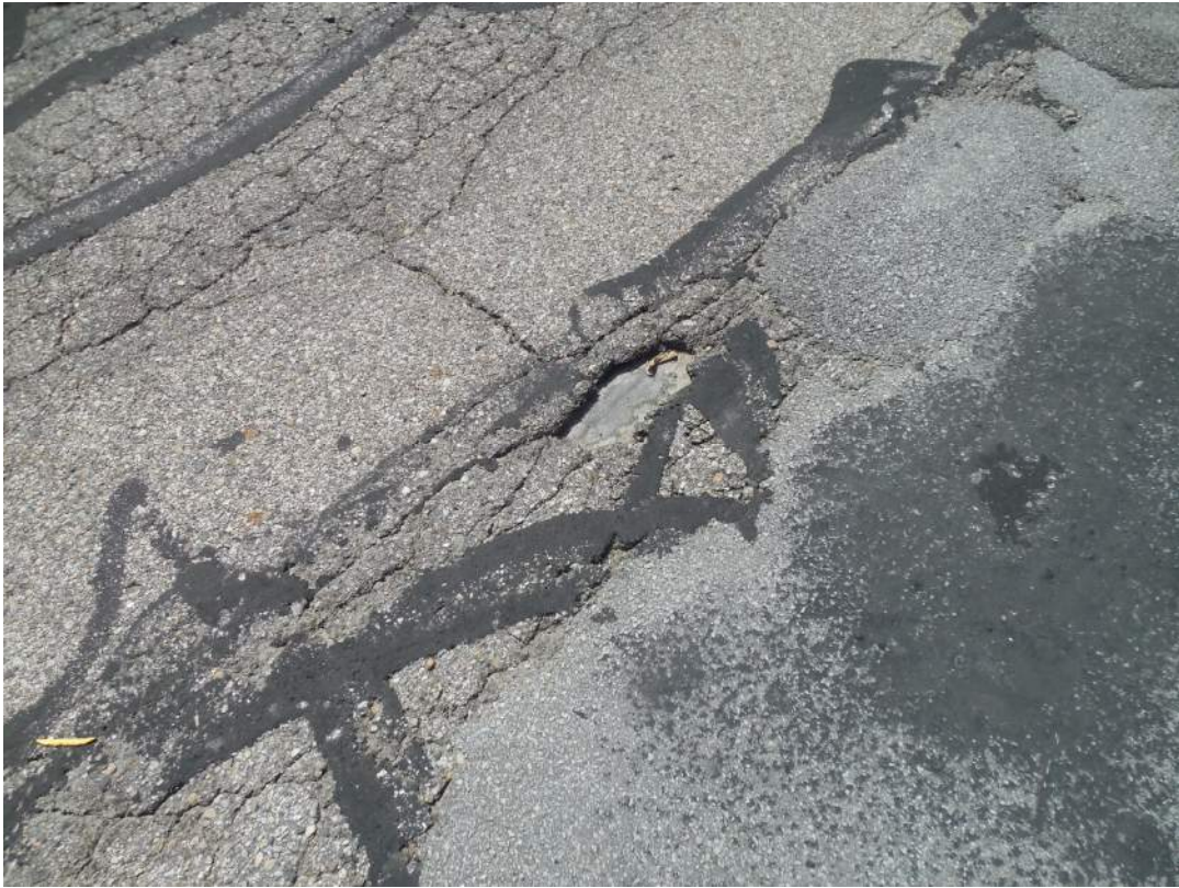
Spalling in asphalt wearing surface with exposed waterproofing membrane
