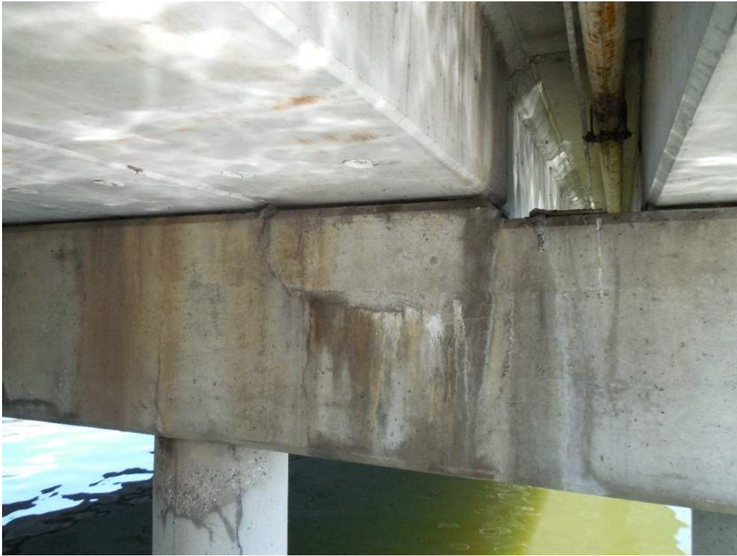
Pier 2S, south face, cracking and delamination at Beam 12W
