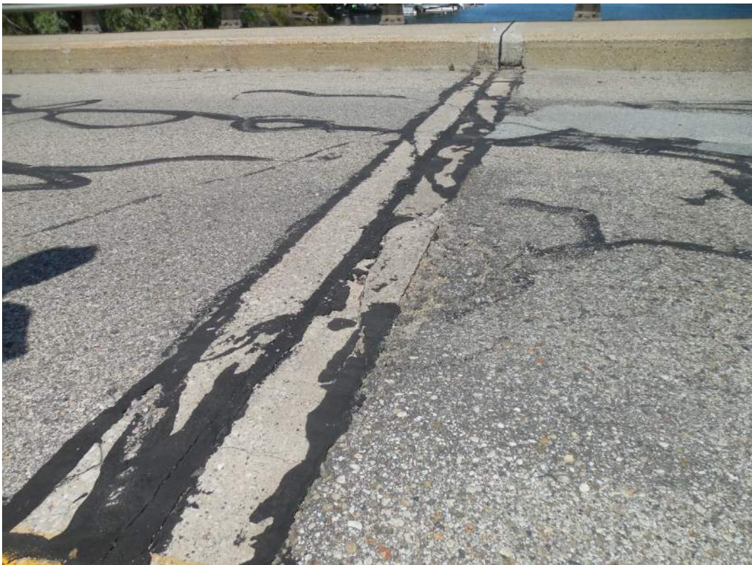
Spalling on expansion joint header in southbound lane
