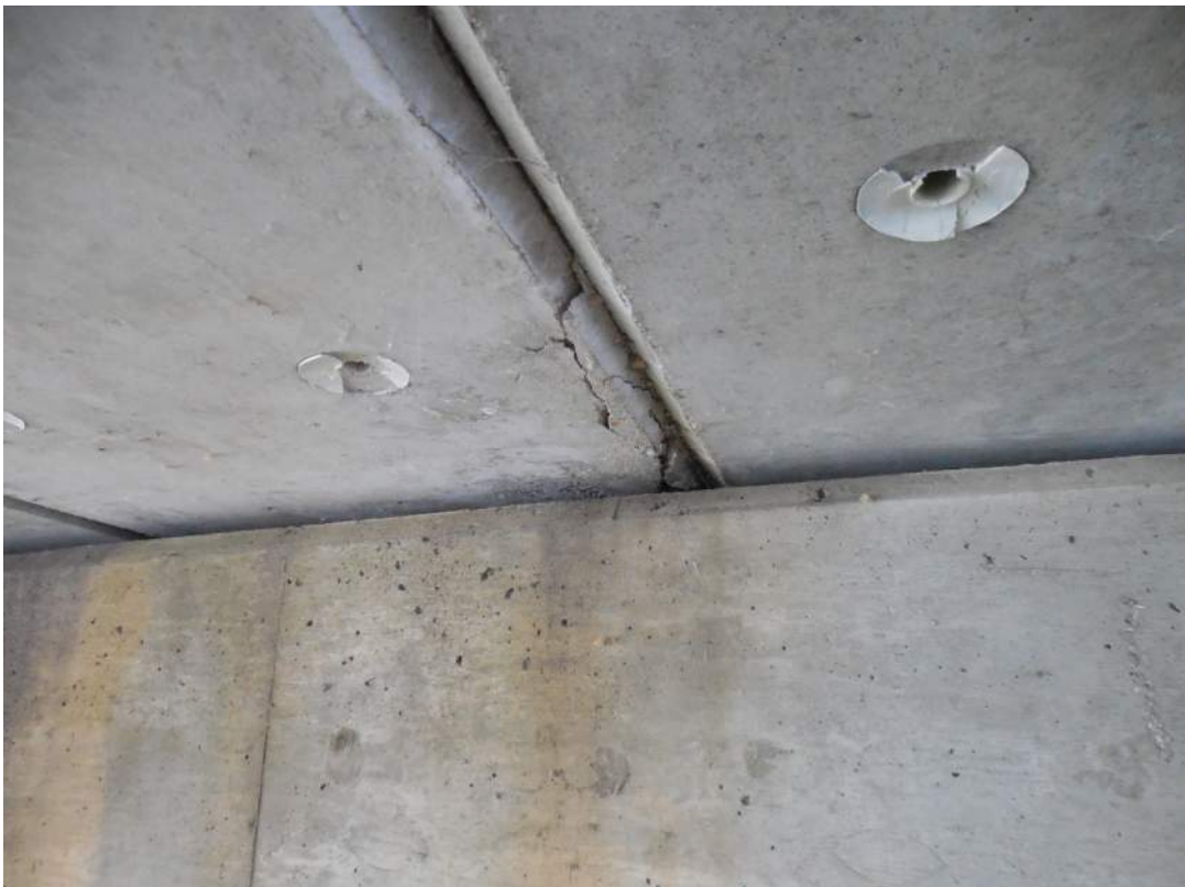
Span 2S, Beam 9W, cracking and delamination at Pier 1S
