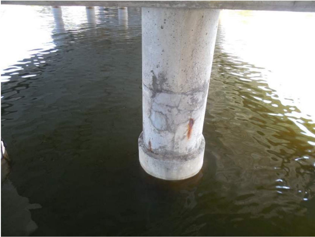
Pier 4S, south face, patching and rust staining on jacket of Pile 4W
