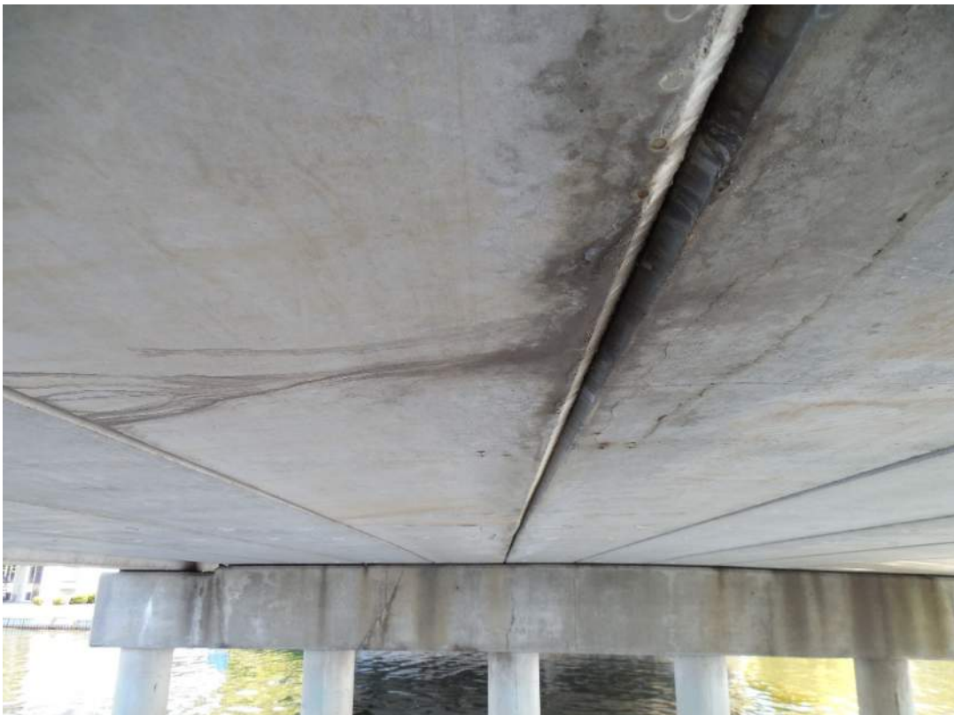
Span 7S, evidence of leakage between Beams 5W and 6W and cracking on 6W near midspan
