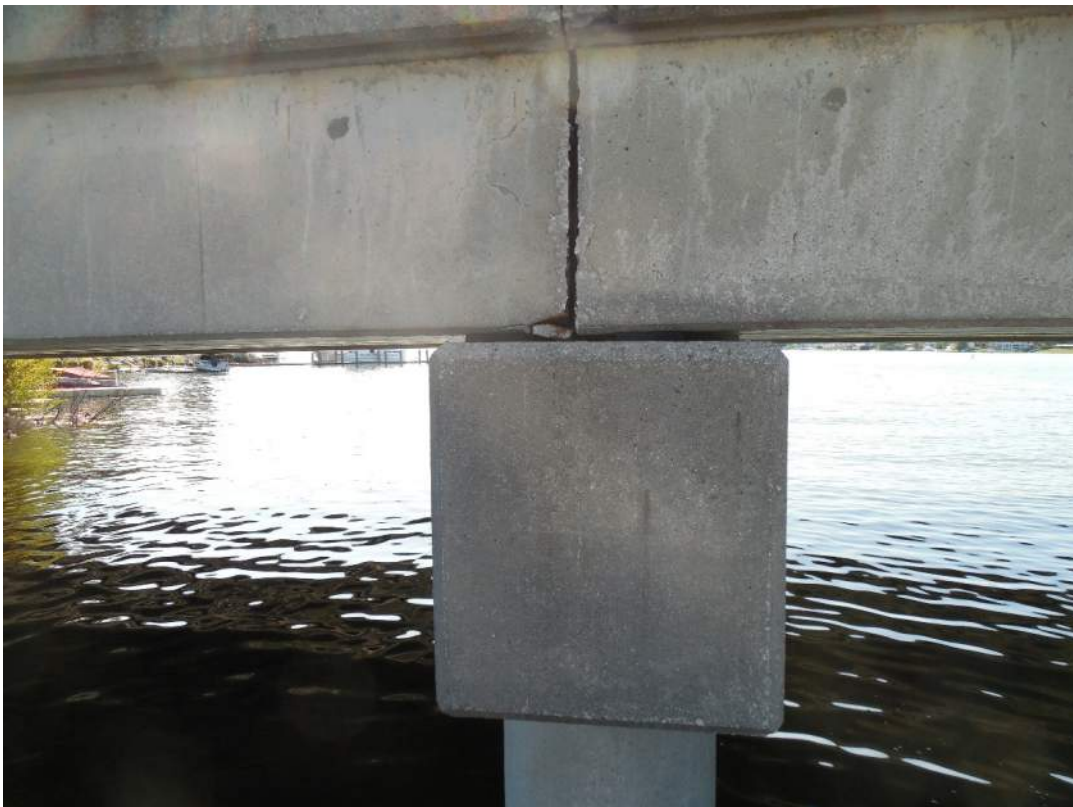
Corner spalling on Beam 1W, Span 8S at Pier 7S
