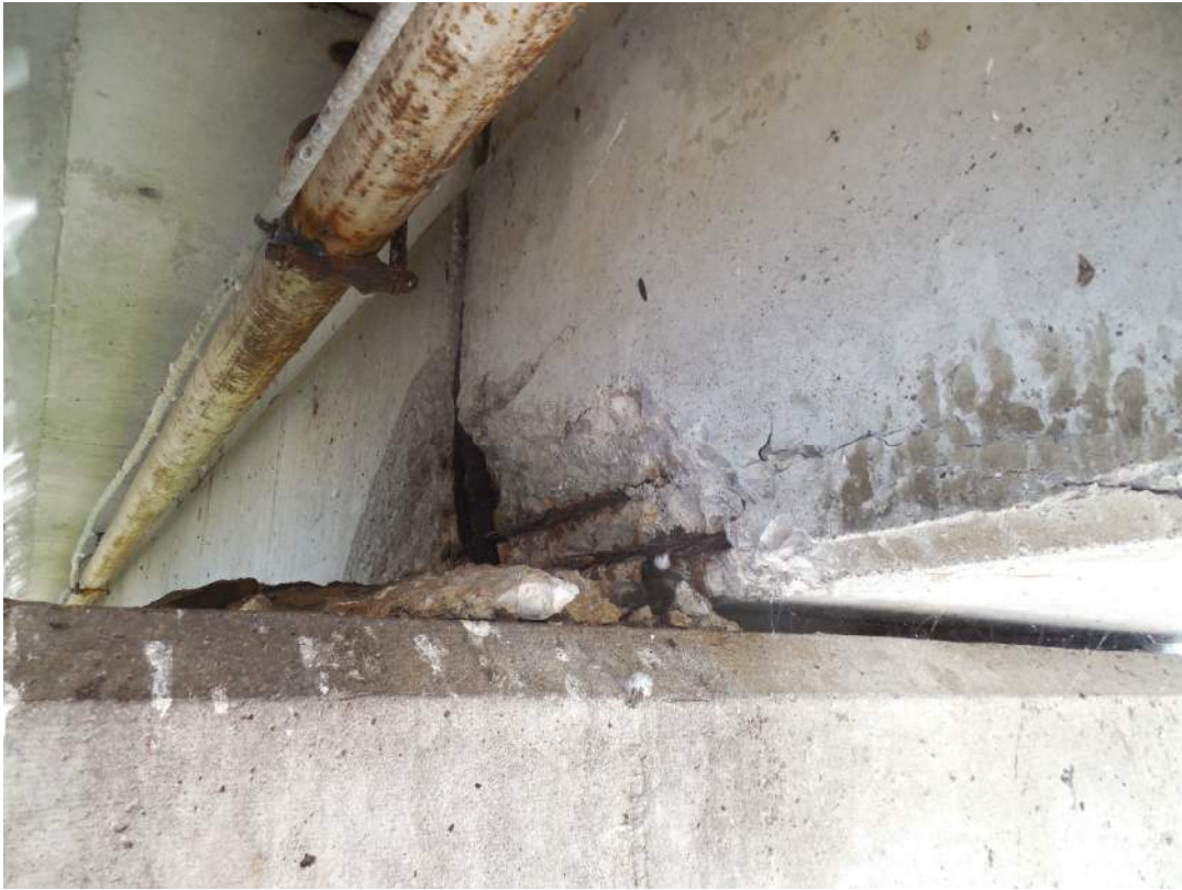
Span 5S, Beam 13W, spalling with exposed steel on interior face at Pier 5S
