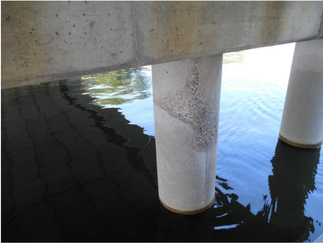
Pier 4S, north face, honeycombing on jacket of Pile 2W
