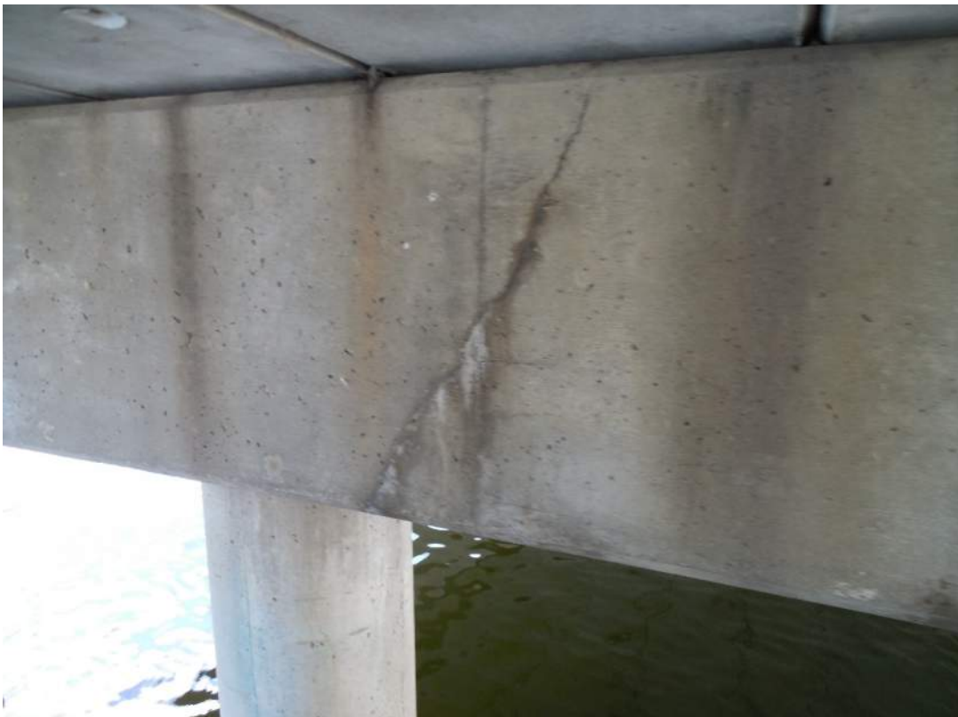
Pier 7S, south face, diagonal cracking with efflorescence on cap at Pile 2W
