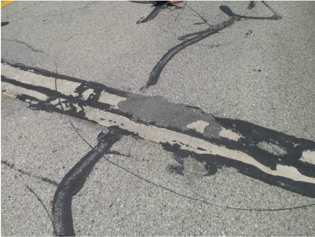
Cold patch on expansion joint header
