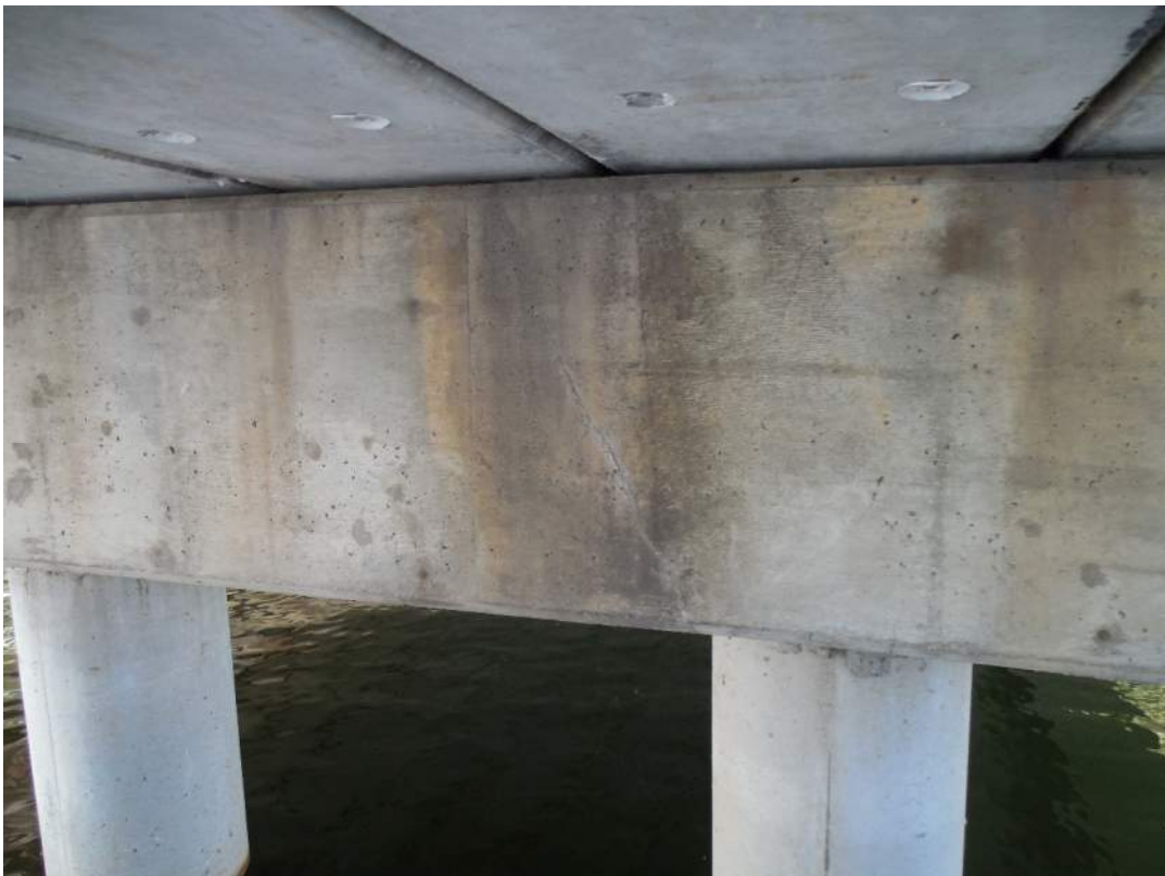
Pier 1S, north face, diagonal cracking at Pile 2W
