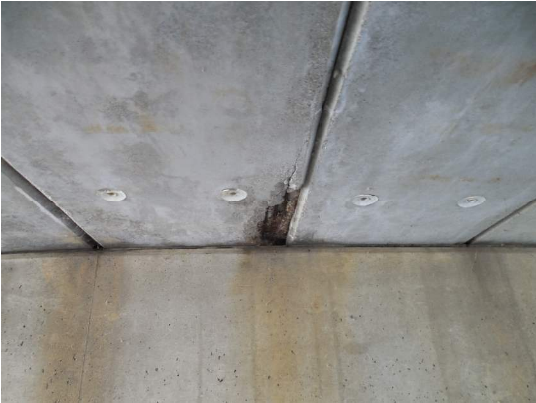
Span 8S, Beam 6W, spalling with 3 broken strands at Pier 7S
