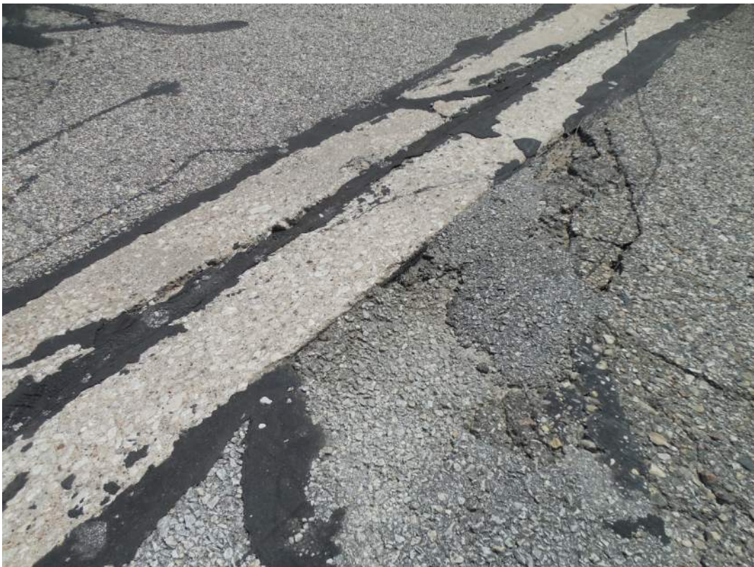
Spalling along expansion joint header and deteriorating joint seal
