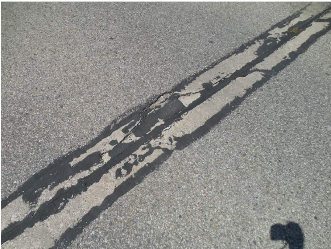
Spalling on expansion joint header
