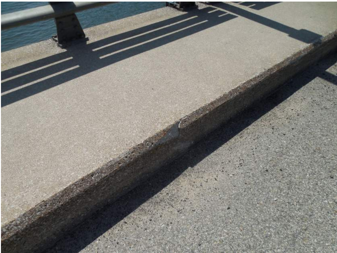
Shallow delamination and edge spalling on east sidewalk
