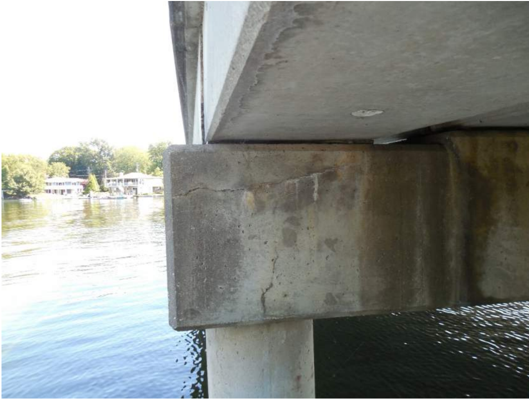
Pier 1S, south face, cracking and delamination at Beam 1W
