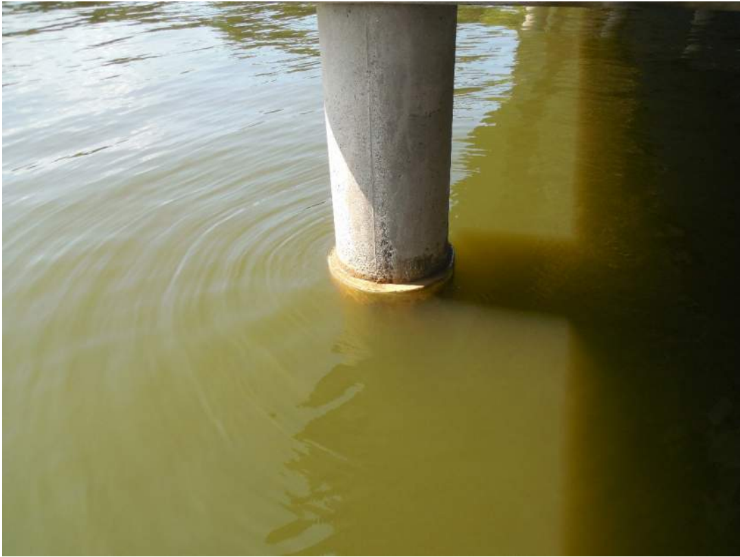
Pier 6S, north face, honeycombing on jacket of Pile 6W
