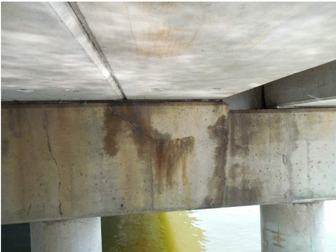
Pier 1S, south face, cracking and delamination at Beam 12W
