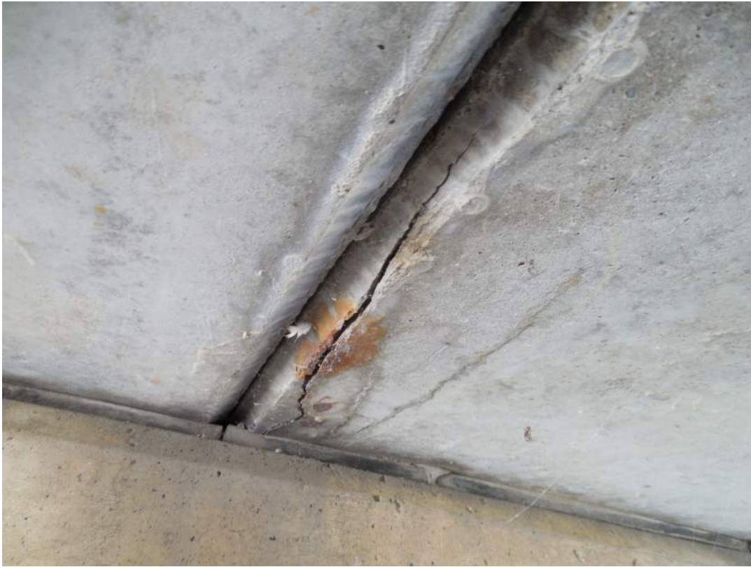
Span 8S, Beam 3W, cracking and delamination at Pier 7S
