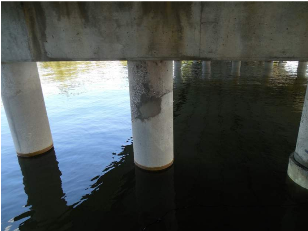
Pier 4S, south face, honeycombing and patching on jacket of Pile 2W
