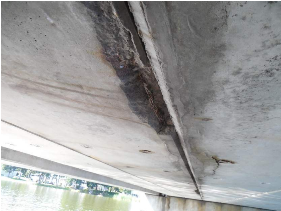
Span 6S, Beam 11W, spalling with broken strand ~15' south of Pier 6S and cracking/delamination on 10W
