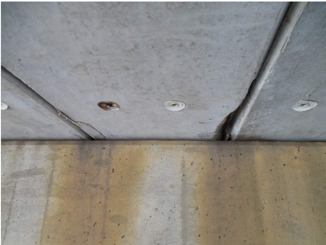
Span 7S, Beam 5W, spalling with broken strand (right) and cracking/delamination (left) at Pier 6S
