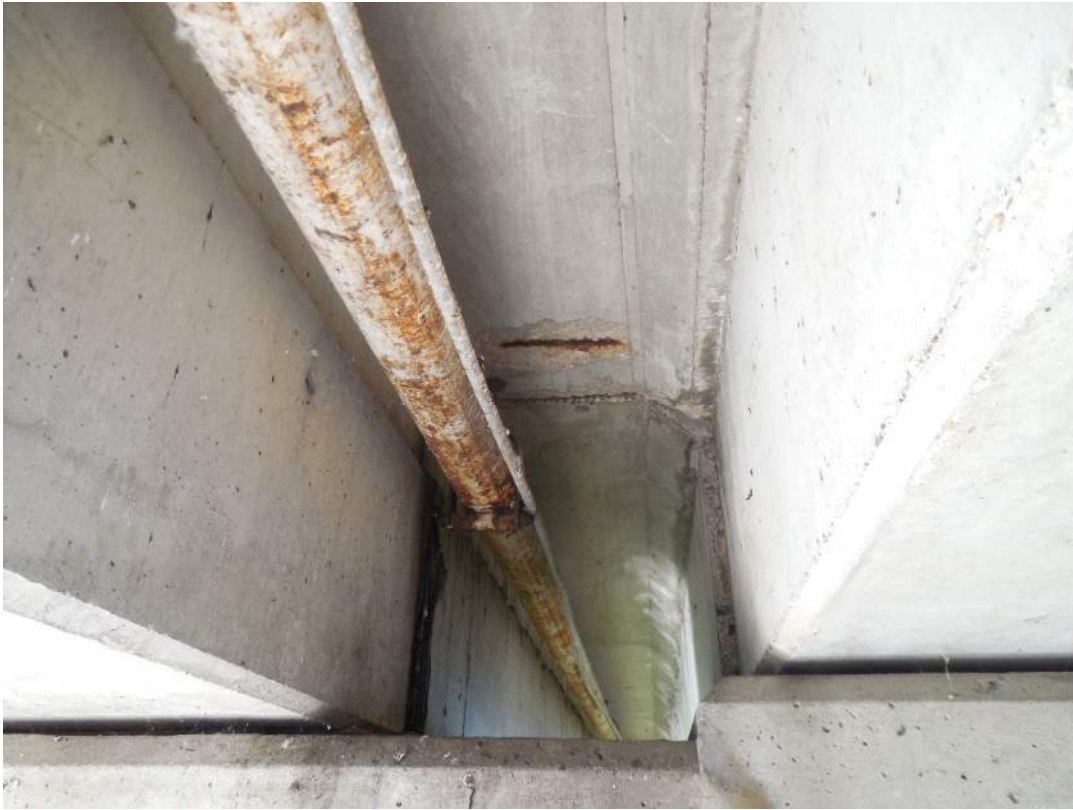
Isolated spall with exposed steel on bottom of sidewalk at Pier 6S
