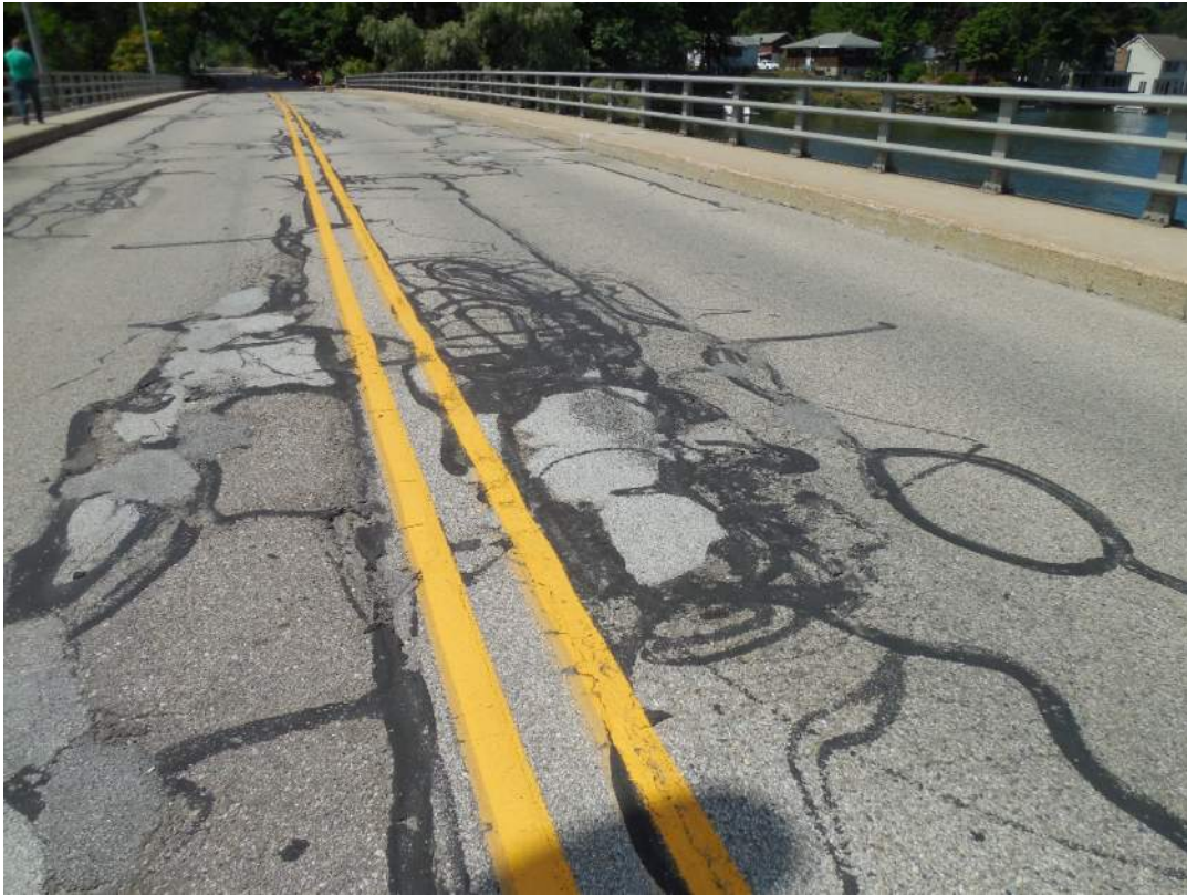
Alligator cracking, spalling and cold patch in southbound lane near center of structure, looking southwest
