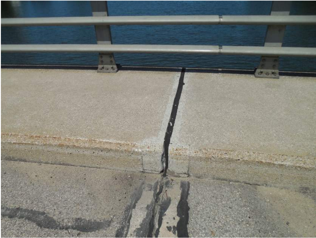
Deteriorating joint seal on sidewalk
