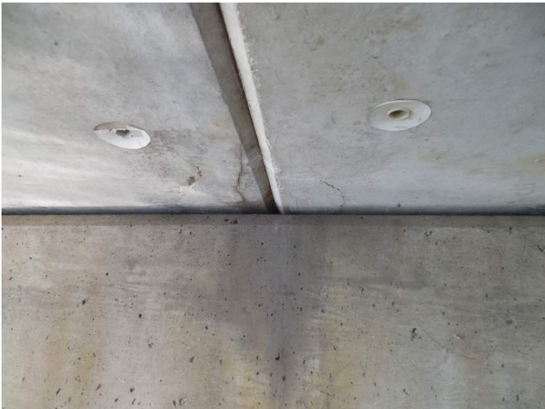
Span 7S, Beams 10W and 11W, cracking and delamination at Pier 6S
