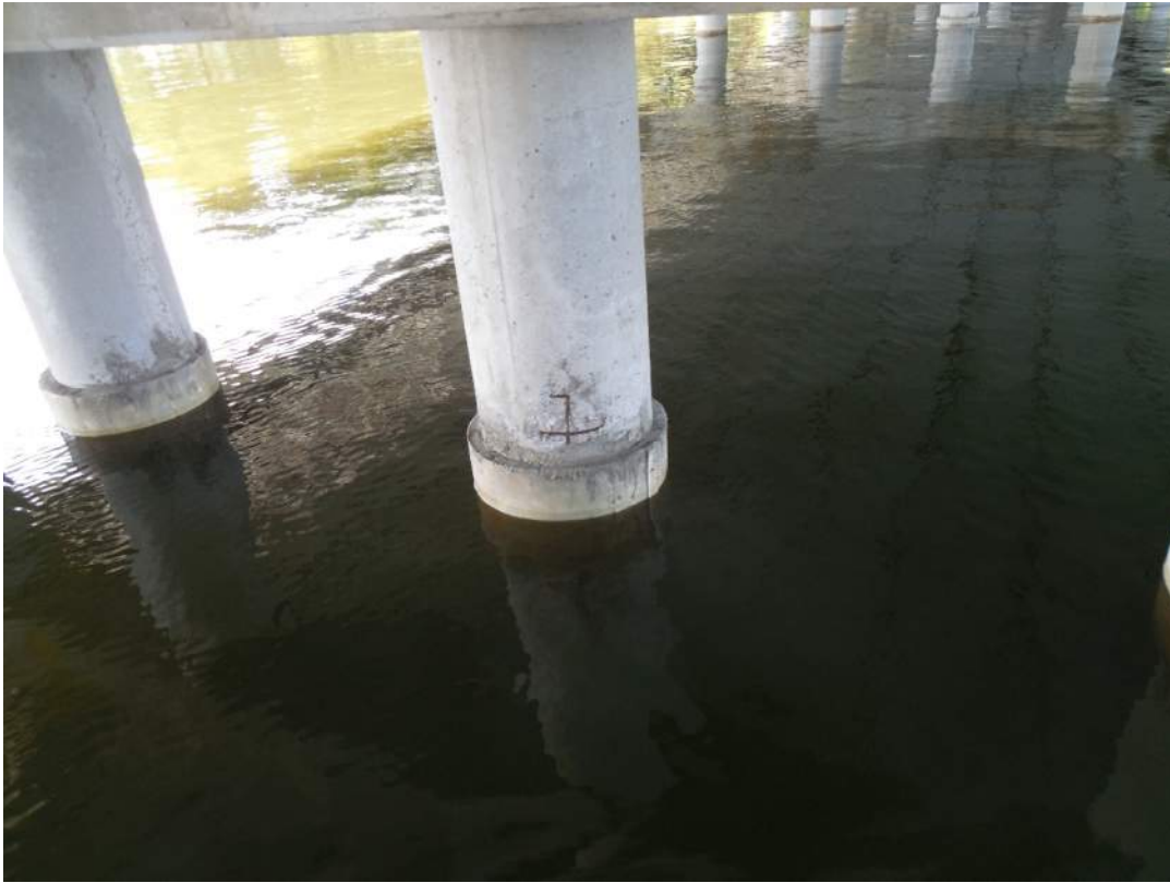
Pier 3S, north face, spalling with exposed steel in jacket of Pile 3W
