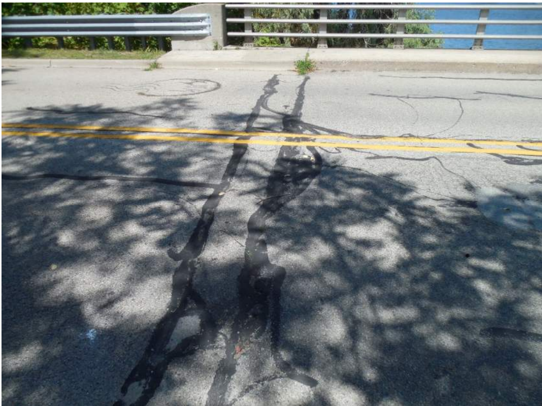
Sealed transverse cracking at south abutment, looking west
