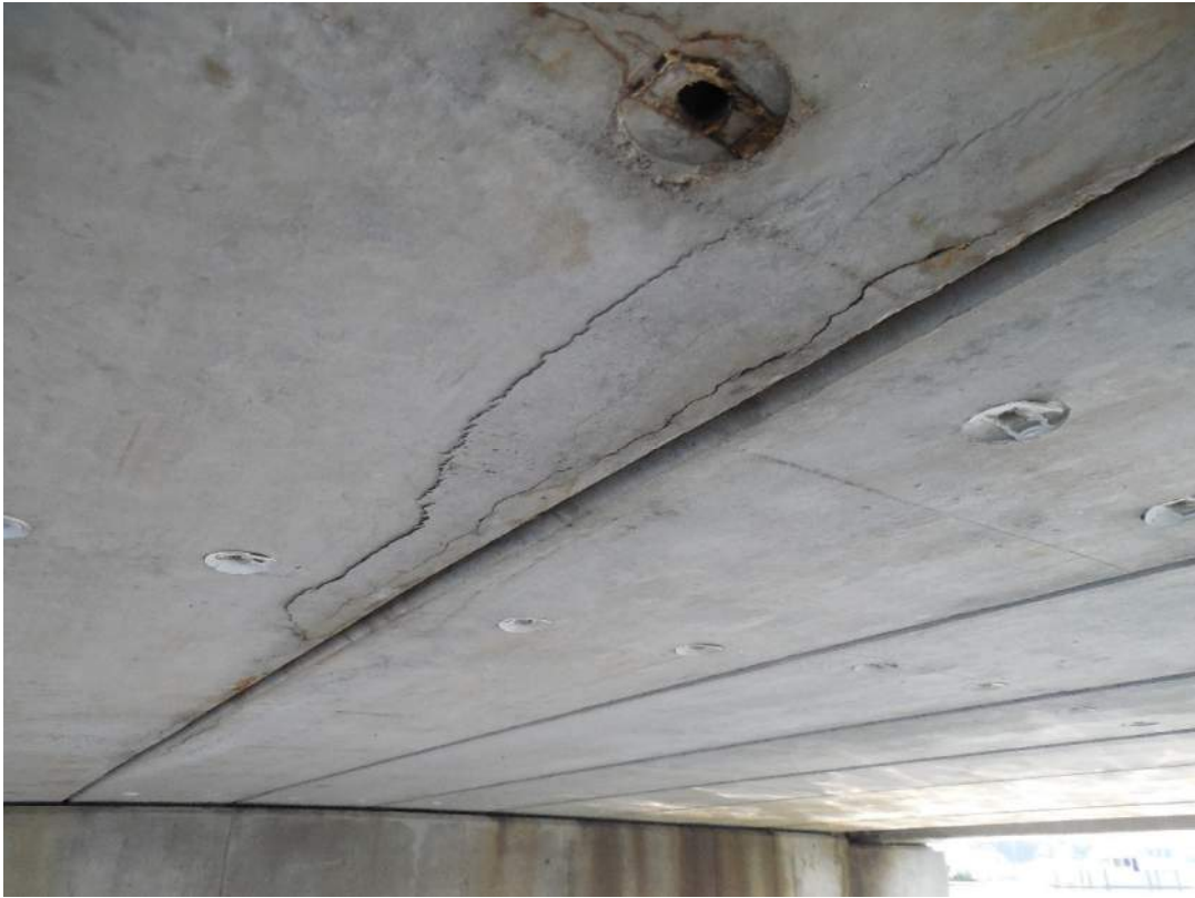
Span 7S, Beam 5W, cracking and delamination north of midspan
