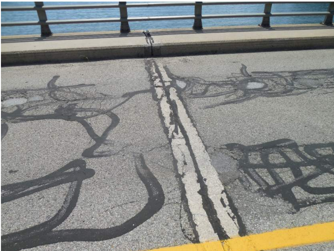
View of expansion joint in northbound lane, south half of structure, looking east
