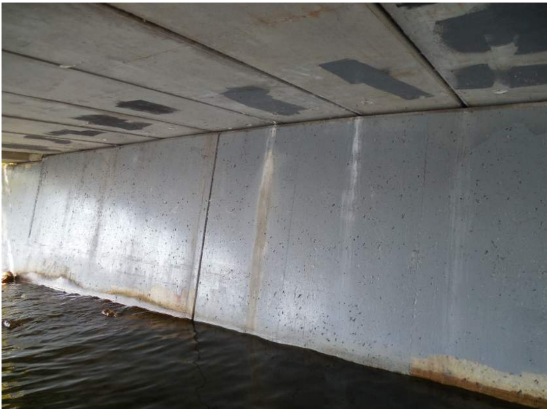
Evidence of leakage at box beam joints on south abutment
