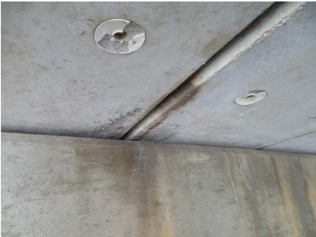
Span 3S, Beam 5W, cracking and delamination at Pier 2S
