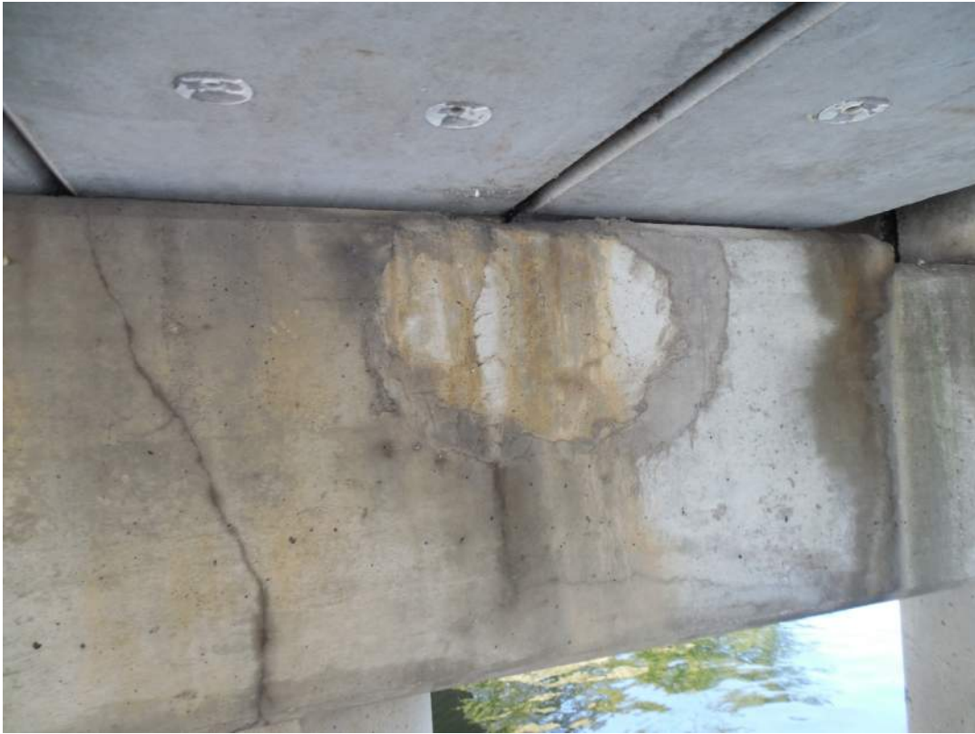
Pier 2S, north face, patched area at Beams 2W and 3W and vertical/diagonal cracking
