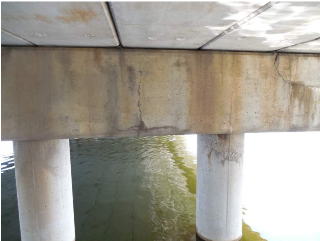
Pier 2S, south face, vertical and map cracking on concrete pile cap, honeycombing on pile jacket
