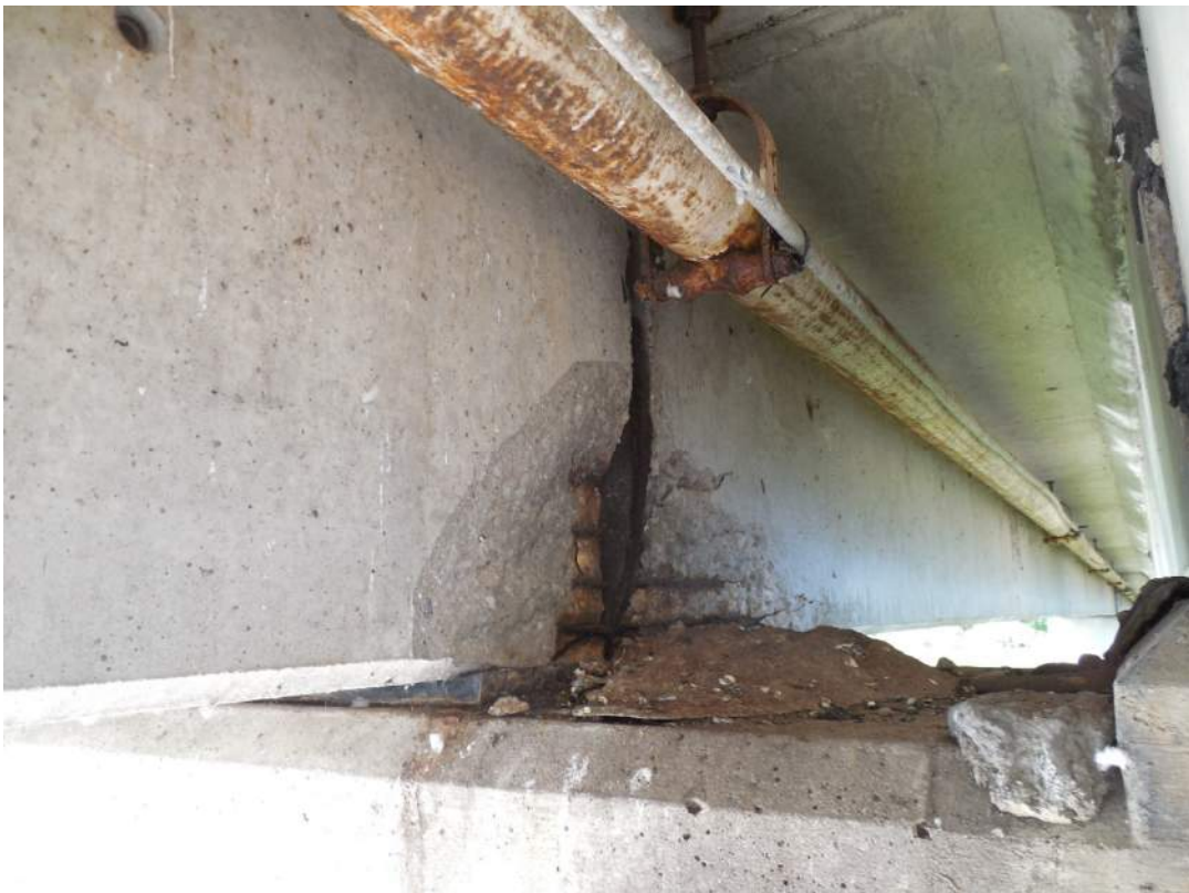
Span 6S, Beam 13W, spalling with exposed steel on inside face at Pier 5S
