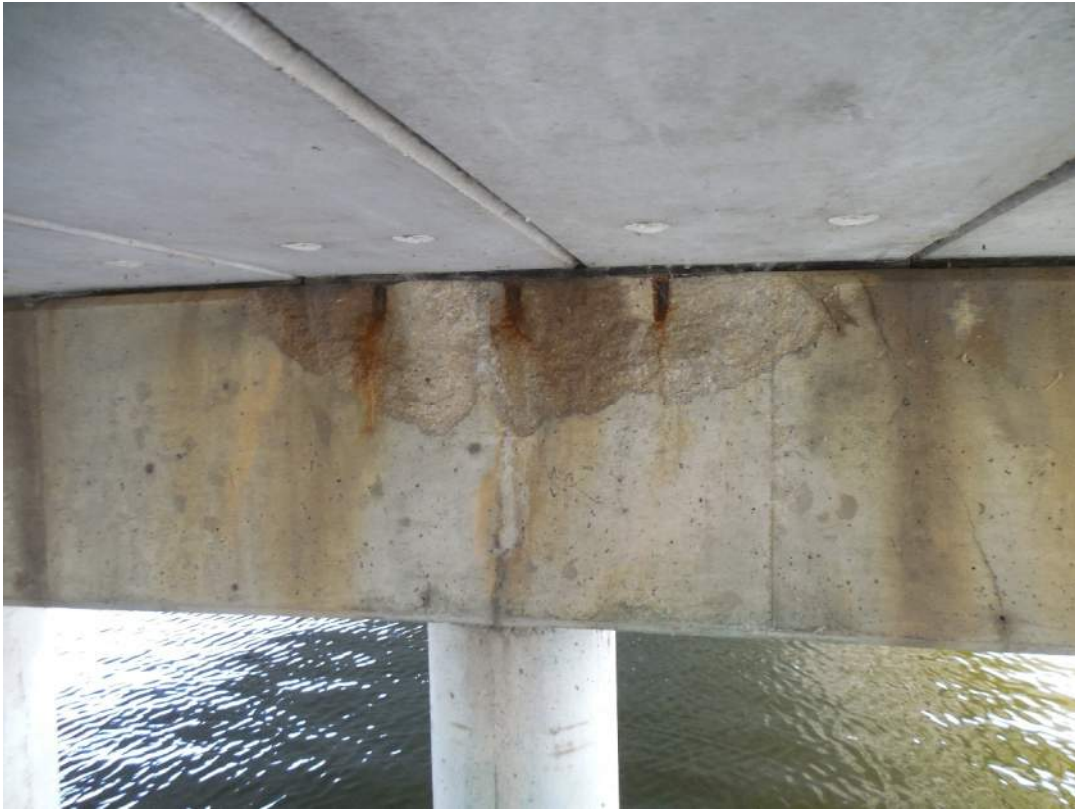
Pier 1S, south face, severe spalling with exposed positioning dowels at Beam 9W
