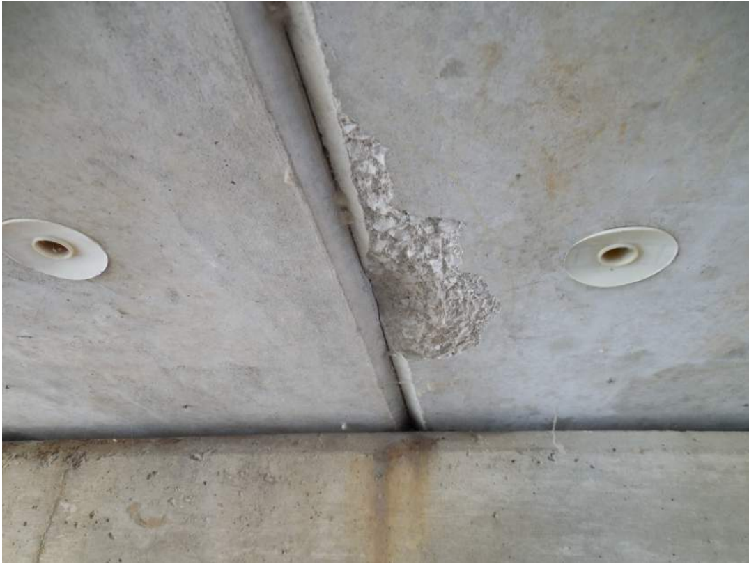
Span 7S, Beam 8W, spalling with no exposed steel near Pier 6S
