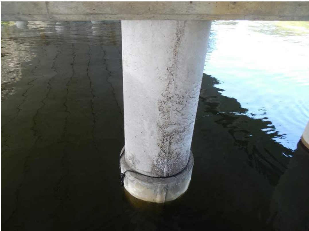
Pier 4S, north face, honeycombing on jacket of Pile 3W
