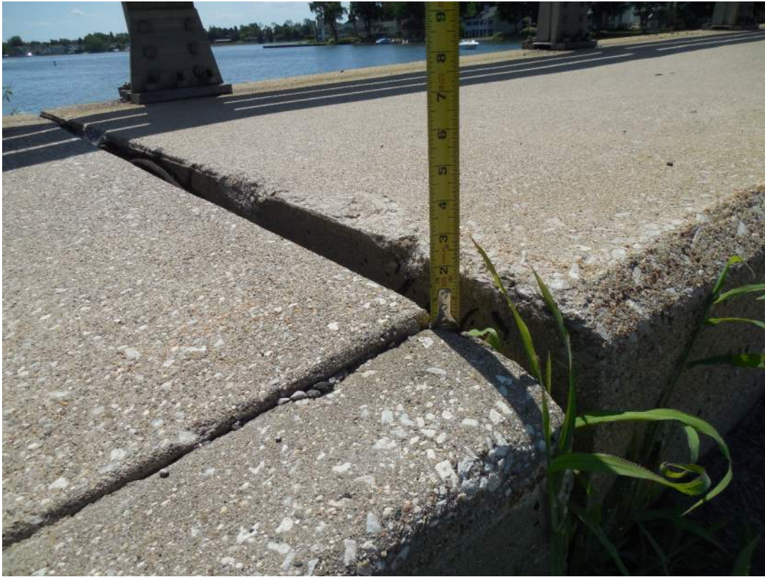
Photo illustrating settlement of northeast approach sidewalk, approximately 2 inches
