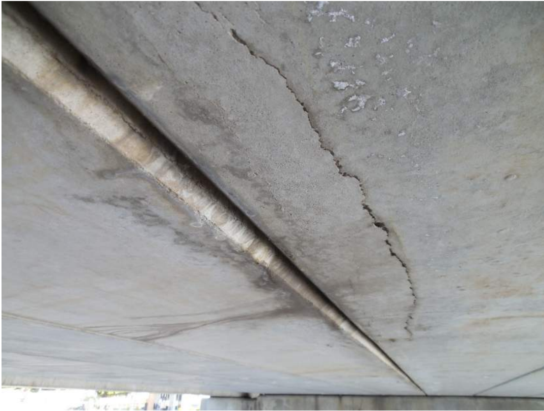
Span 7S, Beam 6W, cracking and delamination near midspan
