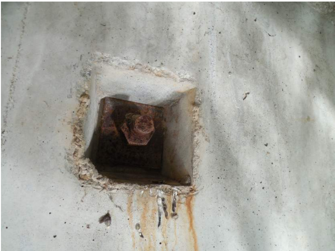
Heavy surface corrosion on post tensioning steel
