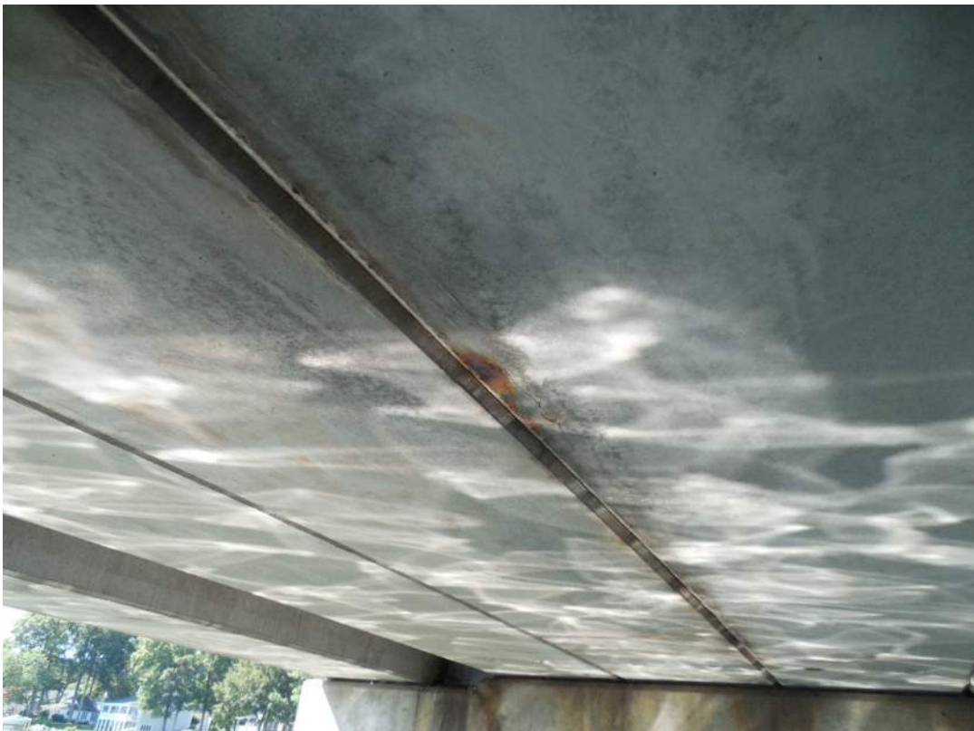
Span 6S, Beam 10W, cracking and rust staining ~15' from Pier 5S
