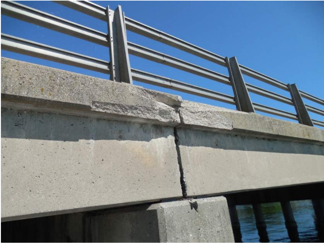
Spalling and grinding on east sidewalk fascia at Pier 2S
