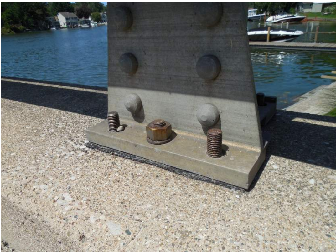
Missing hardware on northwest railing post
