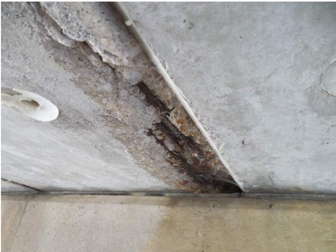
Close-up of spalling at Span 8S, Beam 6W, Pier 7S
