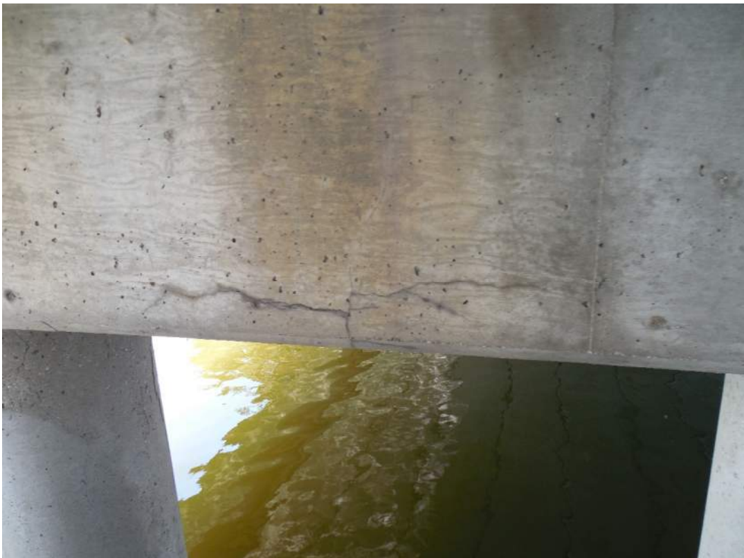
Pier 2S, north face, horizontal/map cracking near bottom of cap between Piles 4W and 5W
