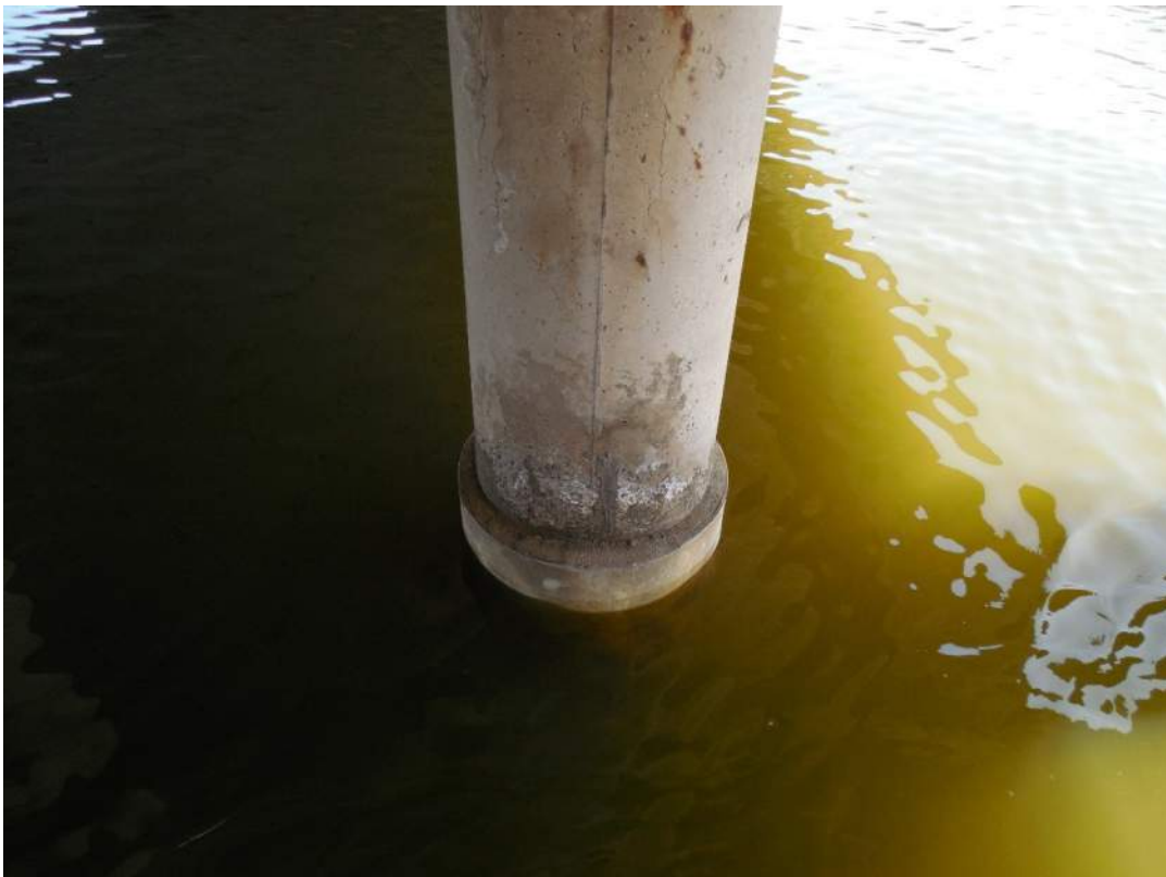
Pier 4S, south face, honeycombing and vertical cracking on jacket of Pile 5W
