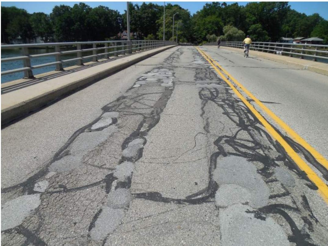
Alligator cracking, spalling and cold patch in northbound wheel lines, north half of structure
