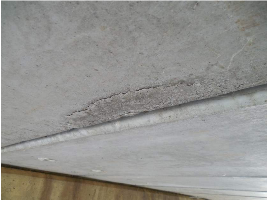
Span 1S, Beam 2W, cracking and delamination ~6' south of Pier 1S
