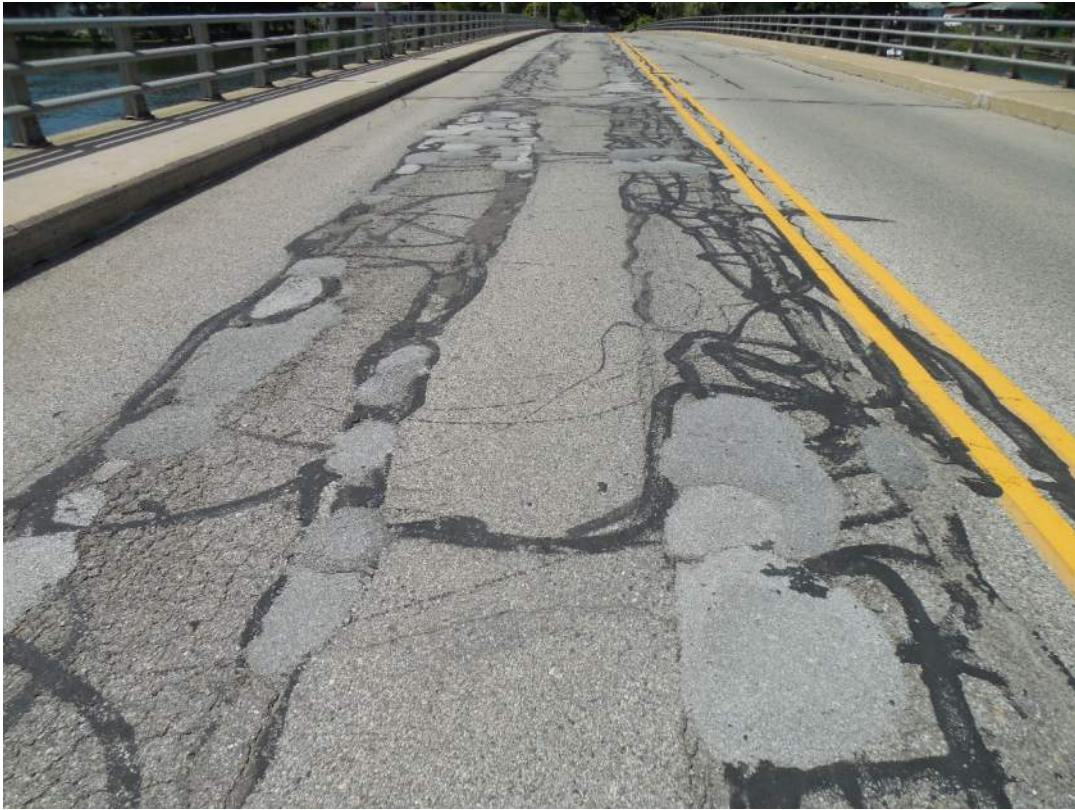
Alligator cracking, spalling and cold patch in northbound wheel lines, north half of structure
