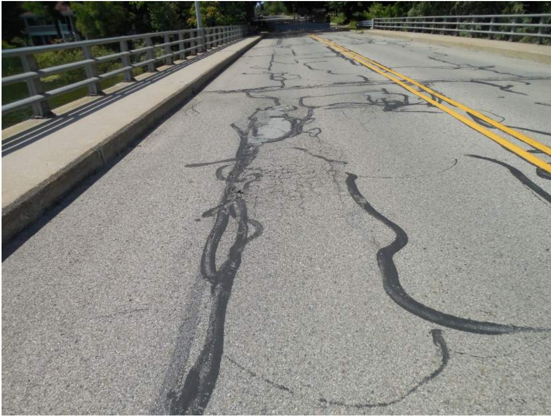
Partially sealed alligator cracking and cold patch in northbound lane, south half of structure, looking south
