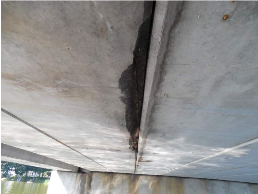
Span 6S, Beam 11W, spalling with broken strand south of midspan
