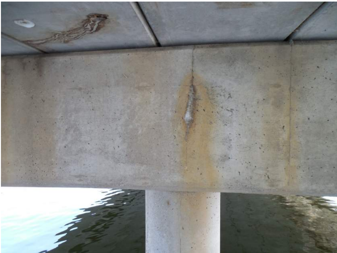
Pier 5S, south face, vertical cracking with efflorescence in cap at Pile 3W
